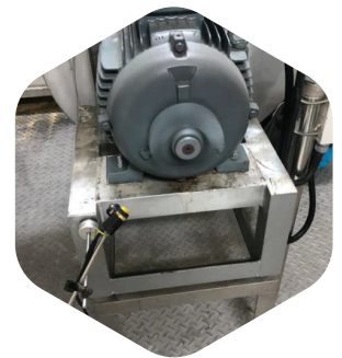
Perform On-Site Balancing For Rotating Equipments
