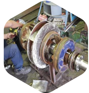
Rotor shaft and impeller balancing facilities
