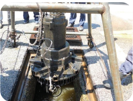
On-site servicing sewage & treatment pumps
